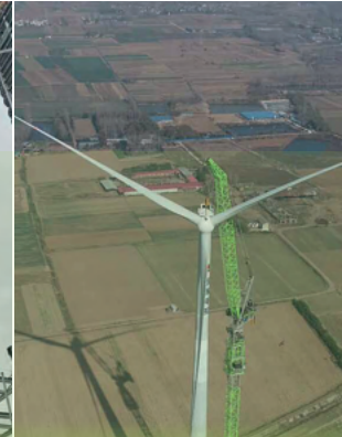
WIND POWER PROJECT / CHINA / LW2340-180
